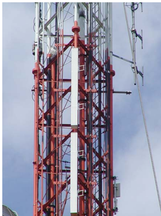
PSI ANTENNA MOUNTED ON THE TOWER. PSI DTV CHANNEL 9 ANTENNA
